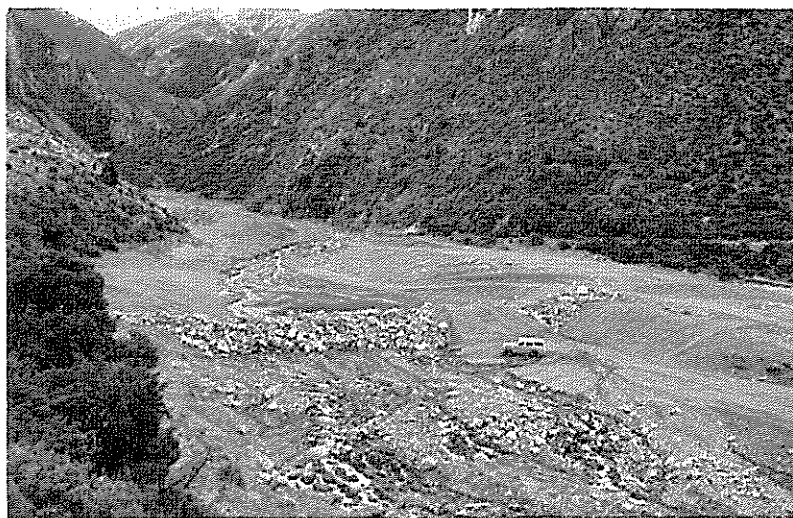
PLATE 2—View from downstream of sediment storage basin, rock dam and platform, Dry Acheron Stream, New Zealand.
